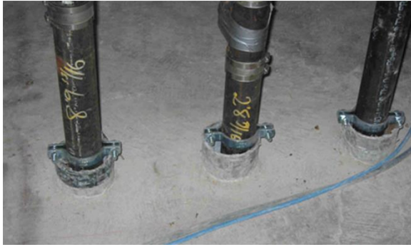
Figure 6: Pipe Going through Floor (© 2007 Iris D. Tommelein. All rights reserved)
