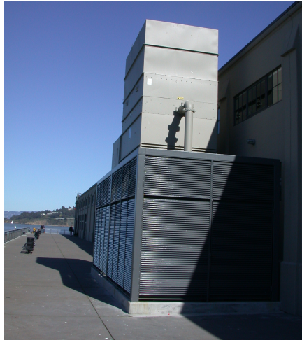
Figure 7.7 Cooling tower Pier 1 (Integral Group 2007).
