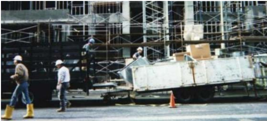
Figure 7: Hand loading of duct segments from delivery truck to trailer that doubles as container for hoisting by crane
